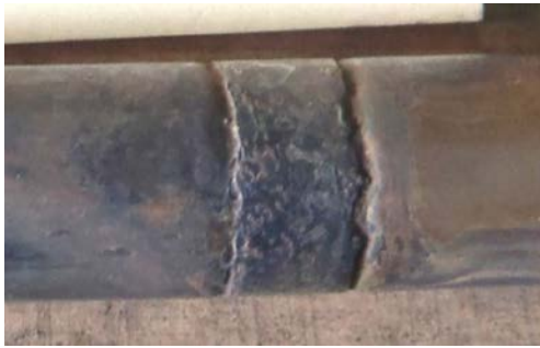
Figure 3. Ammonia grooving of Admiralty brass. This damage occurred with less than 2 years of service.
