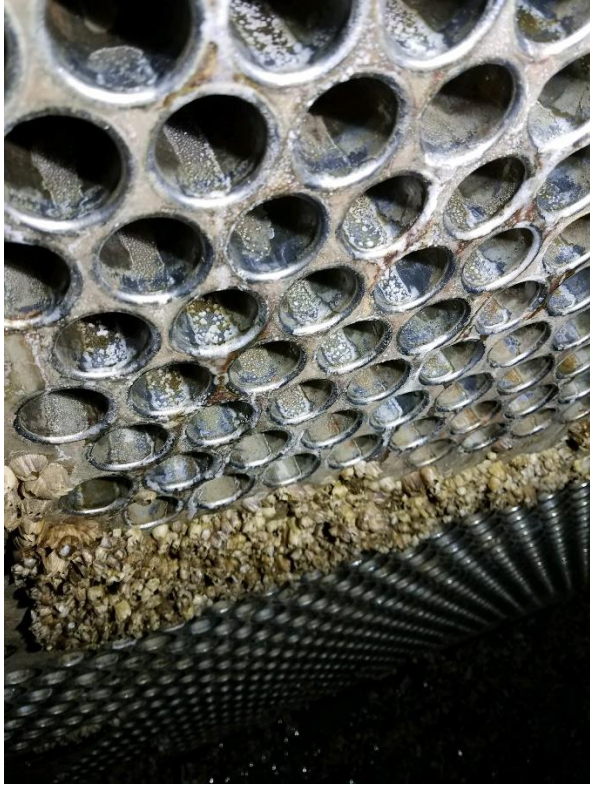
Figure 7. A combination of sea-salt crystals of tubes left to dry at the top and macrofouling at the water level on an improperly laid up seawater condenser bundle.
