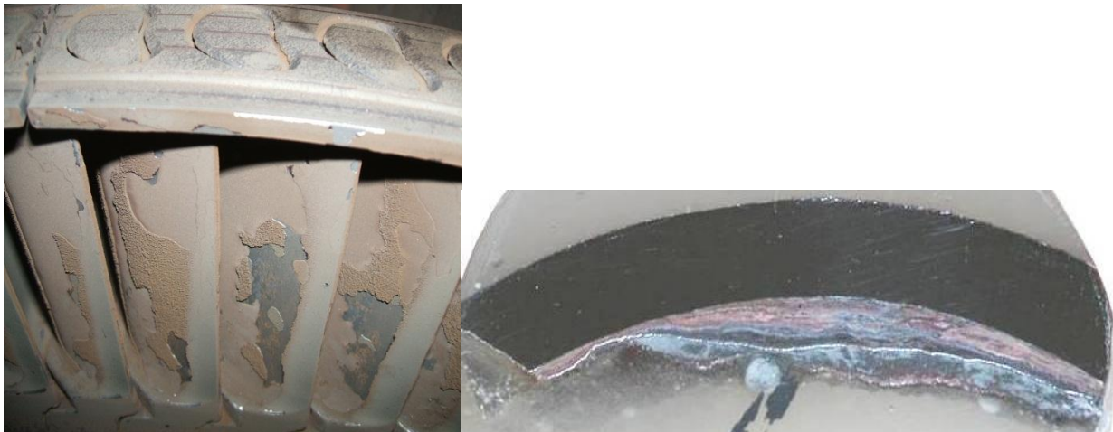
Figure 6. Copper deposits on HP turbine at Pacificcorp Huntington Unit 2 and layered alternating iron and copper deposits on boiler tubes.(ref. 10)
