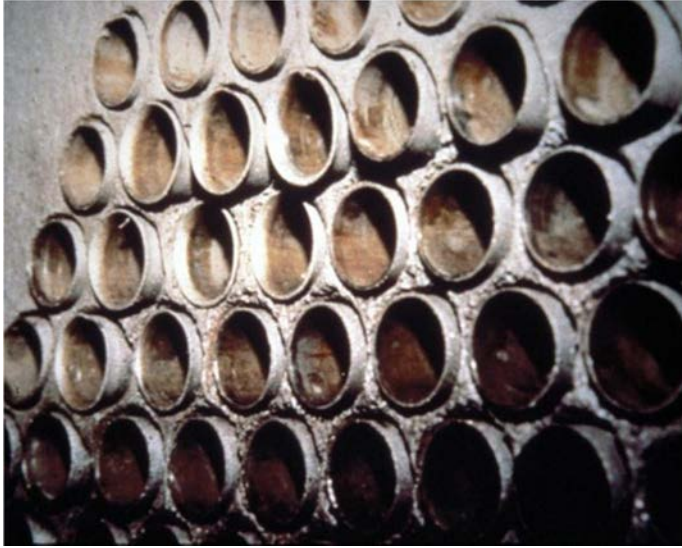
Figure 1. Galvanic attack of a carbon steel tubesheet in contact with stainless steel tubes in high conductivity water (courtesy of Plastocor)
