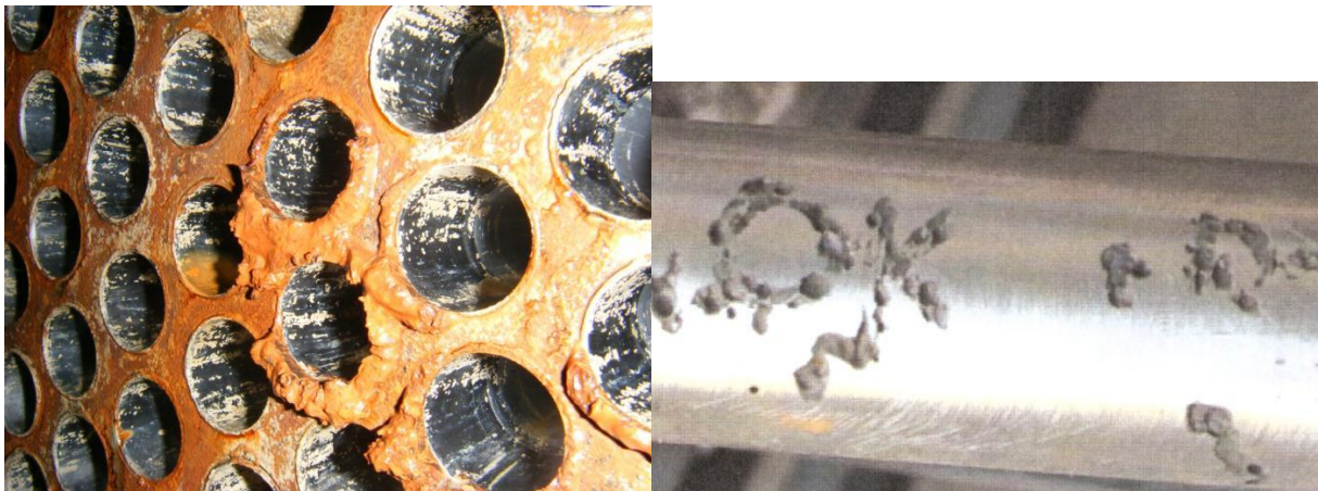
Figure 4. Two examples of unexpected crevice corrosion- the one on the left is of a 321 tube-to-tubesheet joint with S44660 tubes and that on the right is under paint in the shape of OK on a 416 stainless pump shaft
