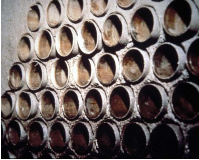
Figure 1. Galvanic attack of a carbon steel tubesheet in contact with stainless steel tubes in high conductivity water (courtesy of Plastocor)
